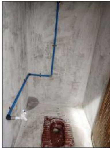
Fig-2 Water Pipeline to the toilet
