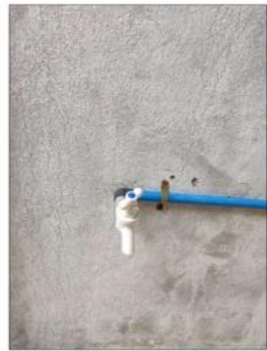
Fig-3 : Water pipe connection to the handwash unit
