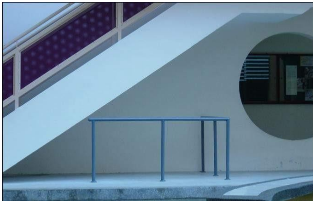
Photo 5.13 Open area under the staircase should be cordoned off
